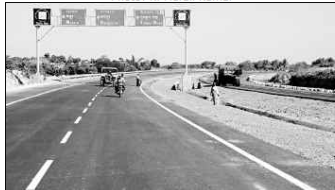
HITS ROADBLOCK: A view of the outer peripheral road connecting Mysore Road and Kanakapura Road, being constructed by Nandi Infrastructure Corridor Enterprise Limited (NICE) as part of Bangalore-Mysore Infrastructure Corridor (BMIC) project.
