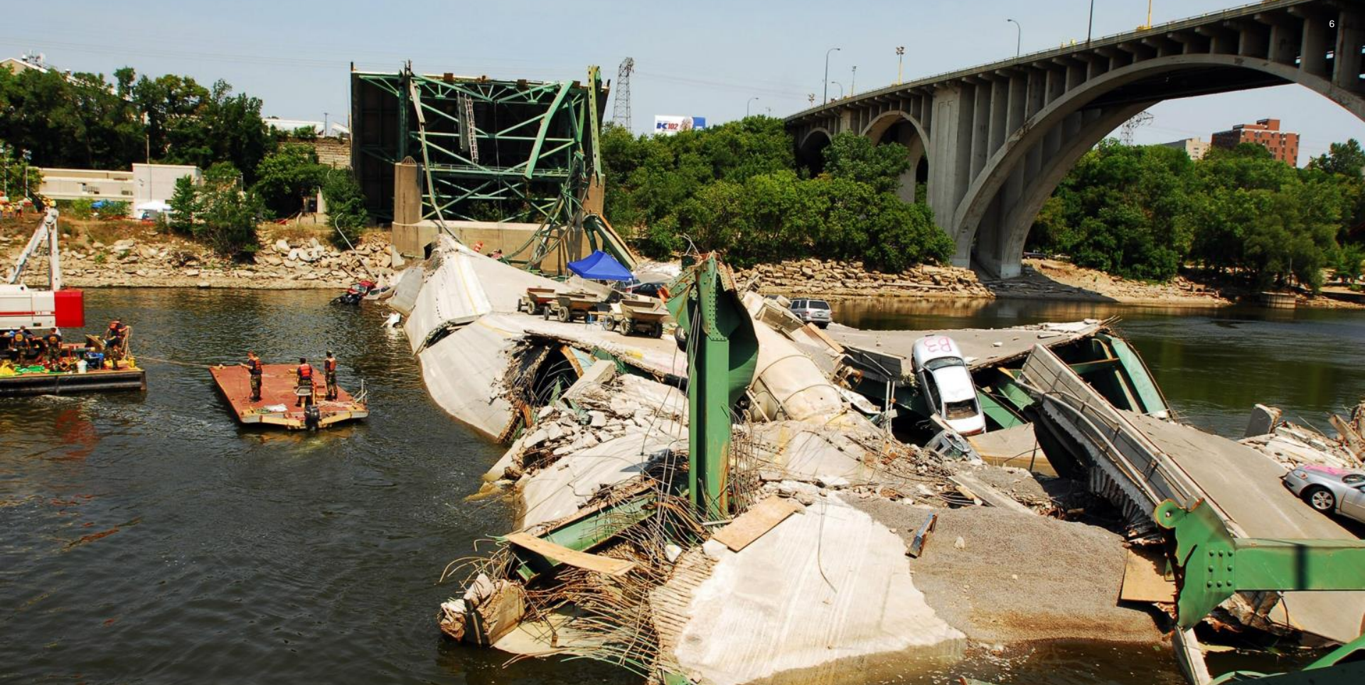
I-35W Mississippi River bridge collapse in Minneapolis, USA
